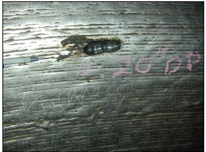
Figure 1. Air-Arc cut gouge for thickness measurement of the overlay by staining with copper sulfate.
