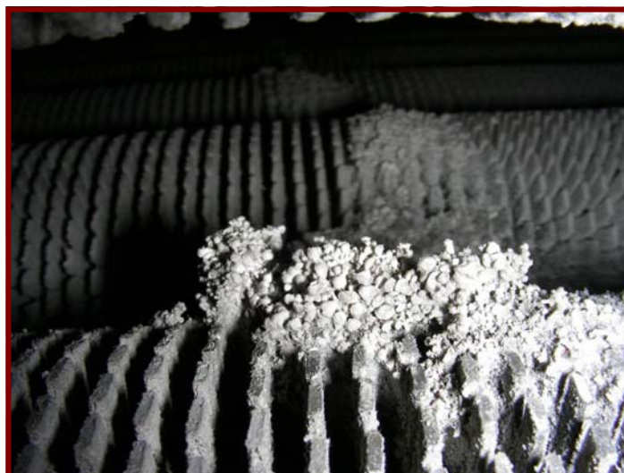
Figure 3. Deposits on the cook water tubes.
