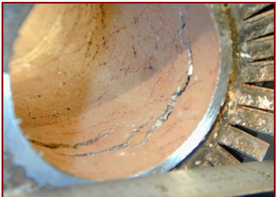
Figure 1. Multiple cracks on this stainless steel feedwater pre-heater tube actually started on the OD of the tube.
