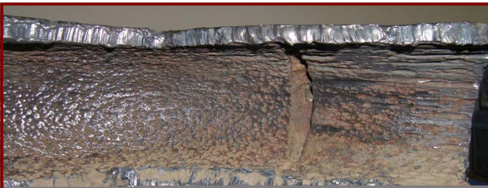
Figure 1. OTSG return pass bend (longitudinal section) showing typical single-phase FAC “orange peel”, along with grooves (merged pits).
