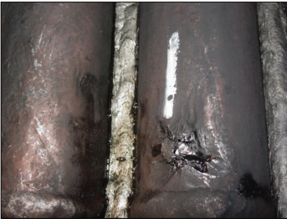
Figure 4. Floor tube leak at weld. The low flow of the horizontal tube combined with weld drop-through initiated DNB boiling tube overheating/thinning.
