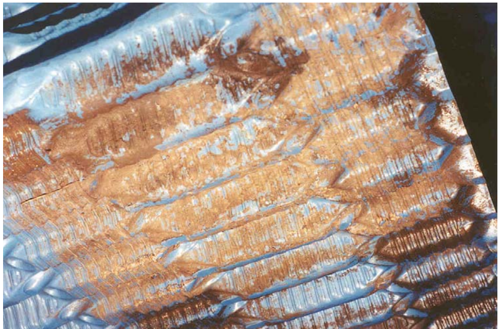
Figure 2. Film fill is an excellent surface area for biofilm accumulation and can be difficult to keep clean.
