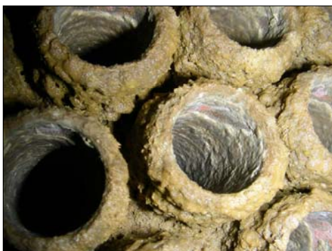
Figure 1. Improper application of biocides can result in biofouling.
