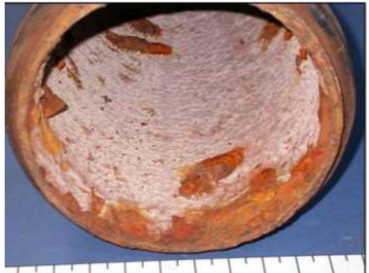
Figure 3. Photograph shows galvanized pipe that was examined after six years in service. This sample was from the cold, softened water line prior to the heat exchanger, but after the circulating hot water return. Pitting was significant.
