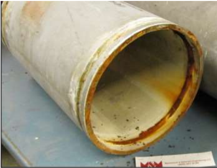
Figure 2. Photograph shows corrosion along a rolled seam at the end of a galvanized pipe
